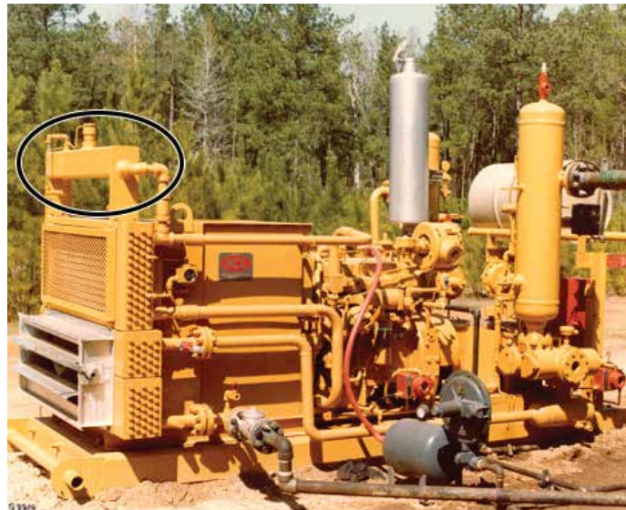
Figure 2.4 — An expansion tank on top of the cooler for a G3304 NA Gas Compressor Engine package. Only one tank is present because the engine is naturally aspirated, which means it will only have the jacket water circuit to cool. The other sections of the cooler are used by the compressor.
