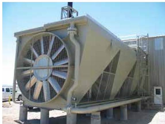
Figure 3.6 — A horizontal cooler on a G3600 Gas Compression Engine installation. Note the multiple stages to support cooling for the engine and the compressor gas.
